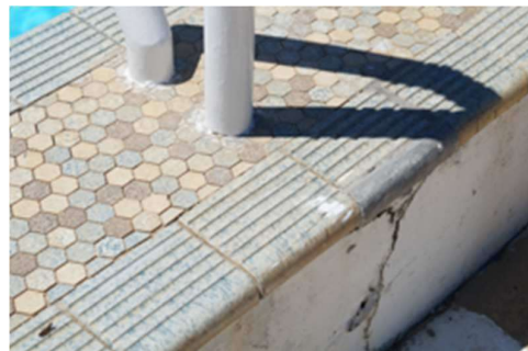
The cracking to the upstand. Cracks runs horizontal along the top and vertical to meet cracking long the concourse paving.
