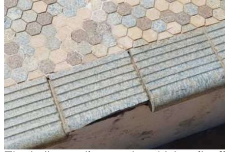
The bullnose tiles cracks which split off.
