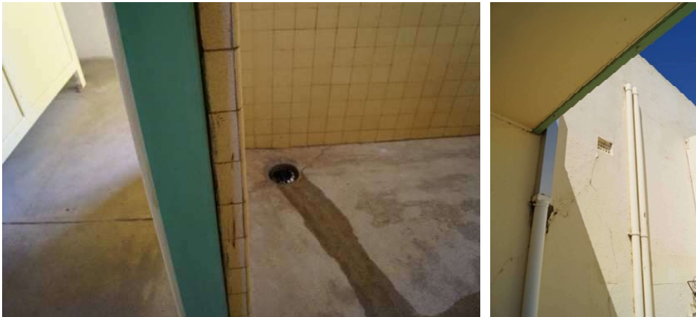
View of the continual water leak in the shower recess in the Men's Changing Room and damage caused to the floor waste. Evidence of both internal and external cracking at the entrance to the Men's Changing Rooms.
