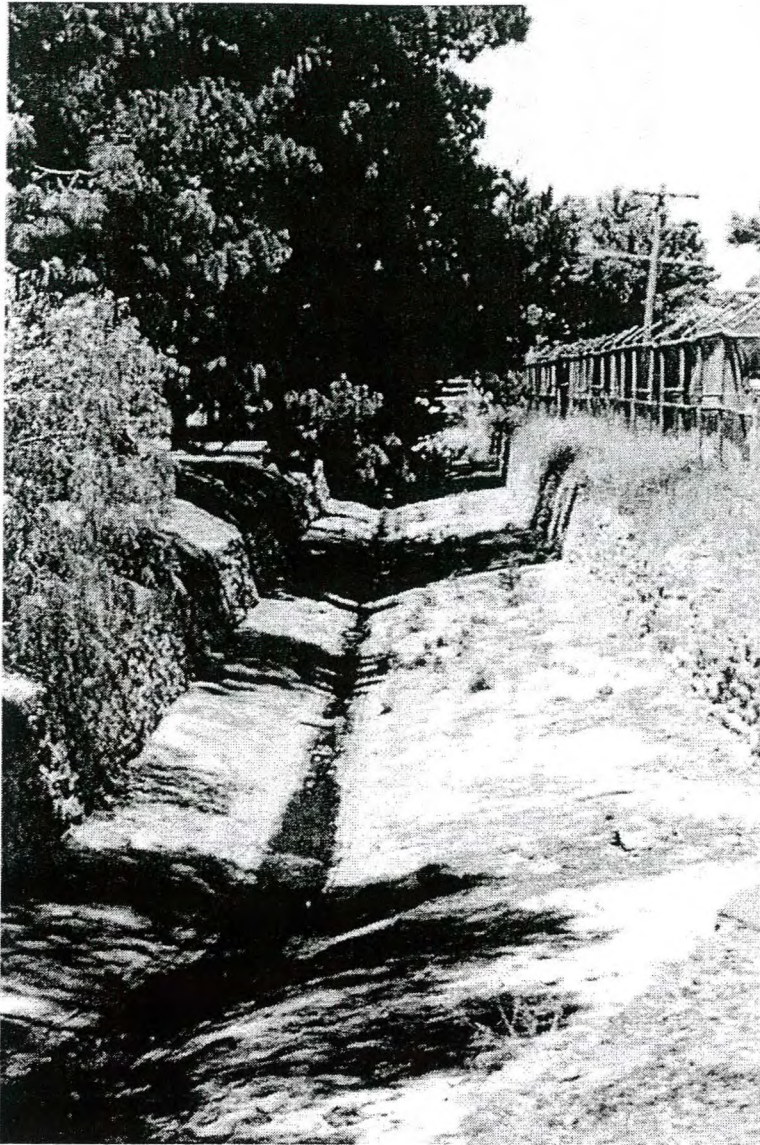
Figure 3.9 Blackman's Lead arm of drain near corner of Alma Street & Earl Street.
