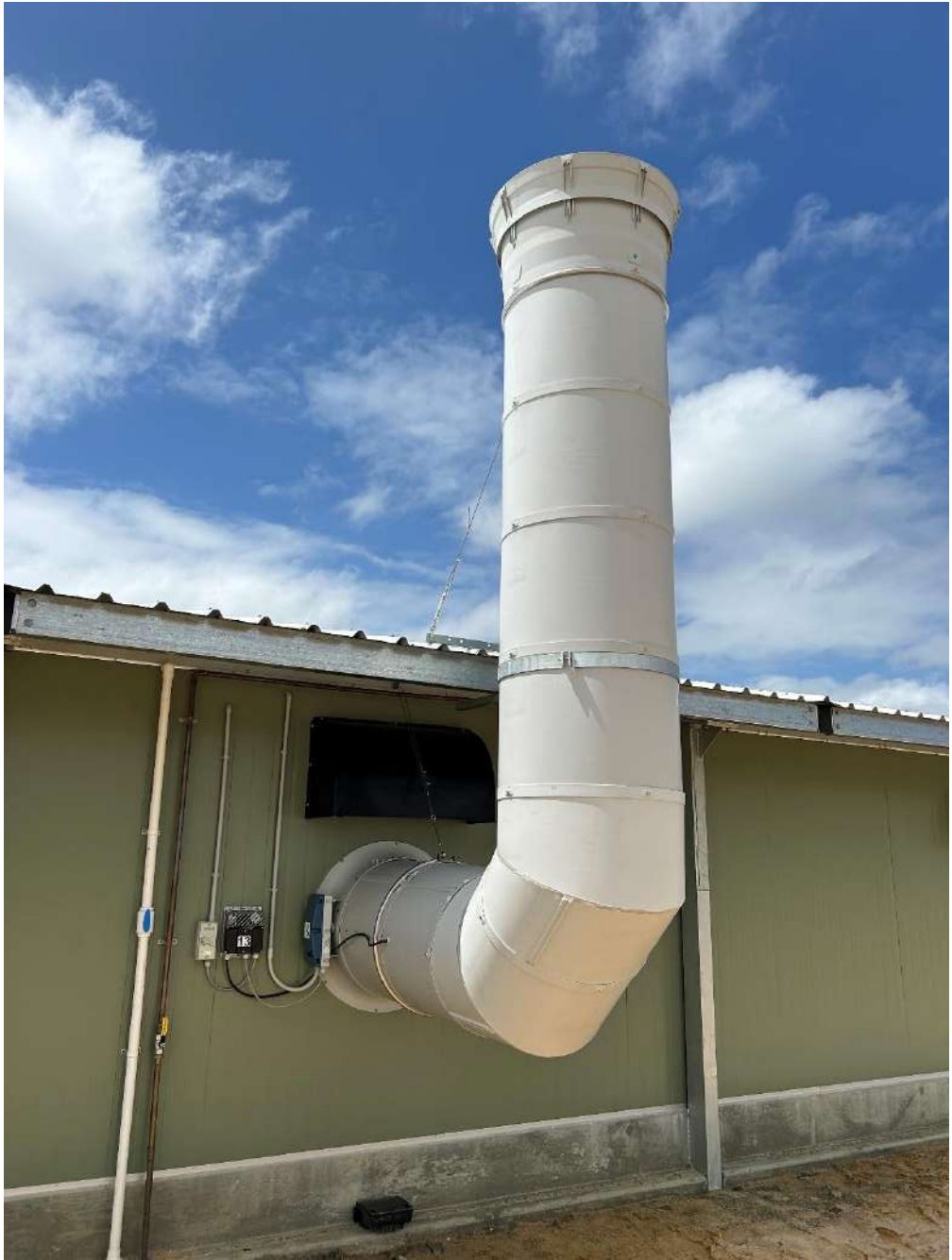
An example of a stub stack
