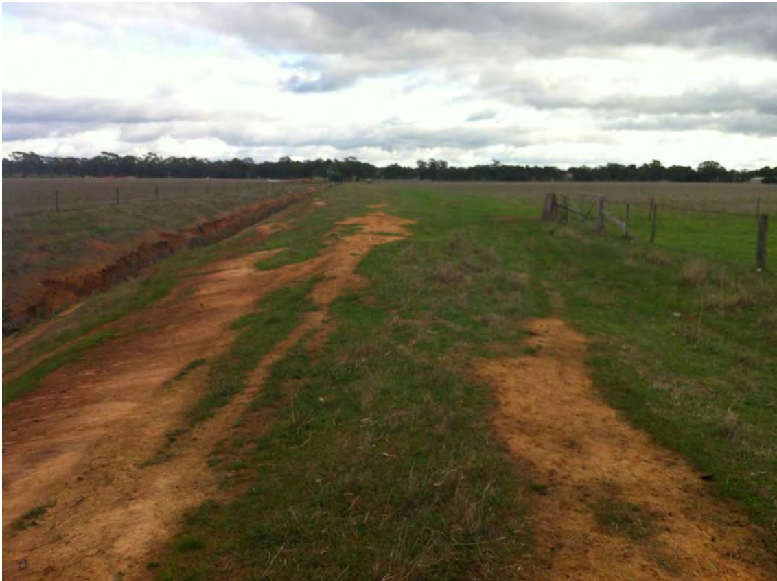
Figure 6. Section of the proposed infrastructure corridor within 200 m of McCallum Creek demonstrating the significant ground disturbance caused by drain construction.
