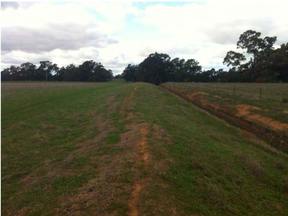
Figure 7. Section of the proposed infrastructure corridor within 200 m of McCallum Creek demonstrating the significant ground disturbance caused by drain construction.
