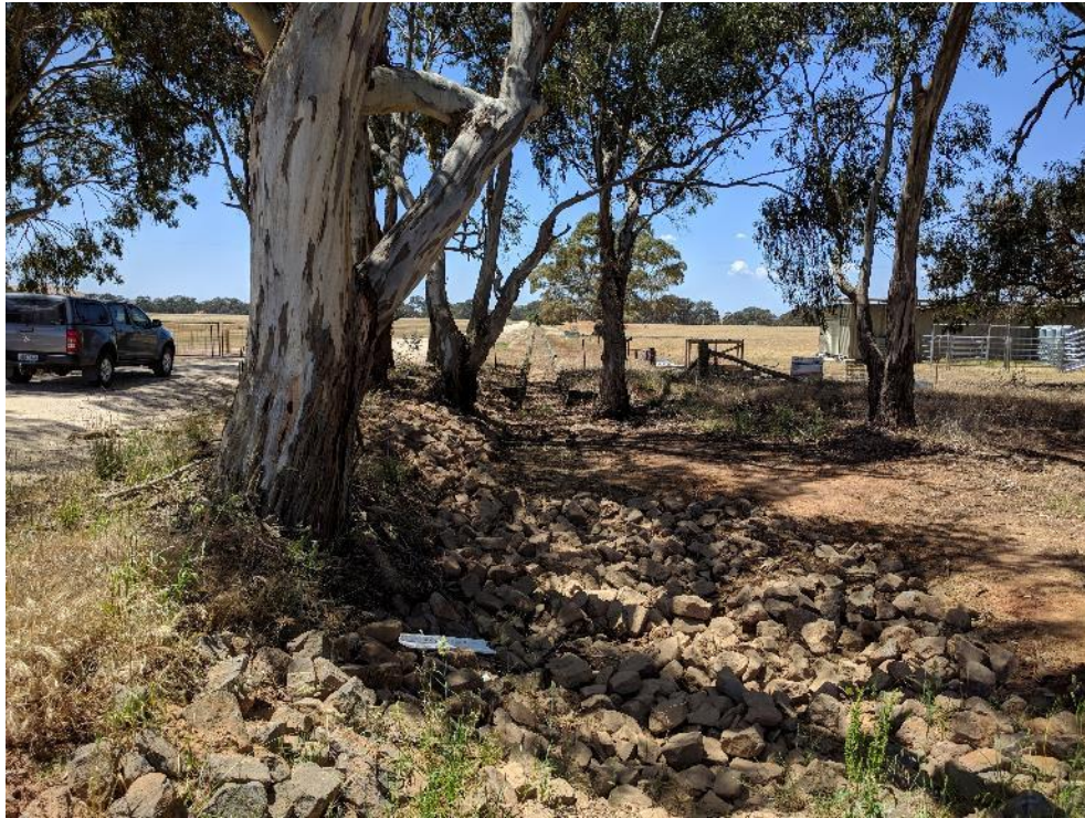
Figure 4.5 : Williams Road Levee and drain at the junction of Williams Road and Landigan Road looking east
