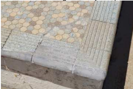
Example of regular repairs to the bullnose tiles using concrete to form the original shape.
