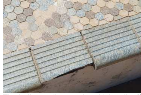
The bullnose tiles cracks which split off.
