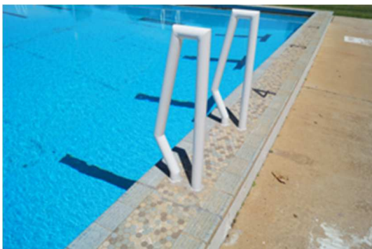
View showing the cracking along the junction of the upstand at the base and also beneath the tiles. Cracks are across the tiles and vertical.
