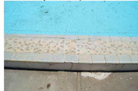
There is evidence of both horizontal cracking and vertical cracking to over 75% of the tiling. This corresponds to widespread horizontal and vertical cracking to the upstand kerb around the pool where the reinforced bars have deteriorated, causing damage.
