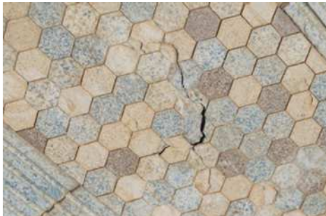
The hexagonal tiles are made of two different thicknesses, where there has been collapse of the substrata due to erosion by water there is irregular cracking through the hexagonal tiles as the thinner tiles settle unevenly. The mortar joints around the tiles are regularly repaired but by summers end are eroded again.
