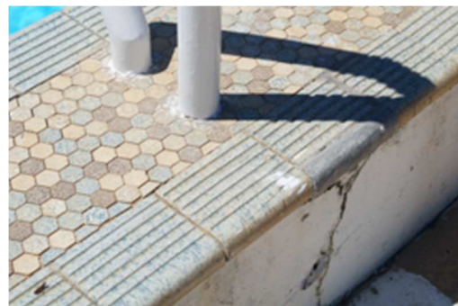
The cracking to the upstand. Cracks runs horizontal along the top and vertical to meet cracking long the concourse paving.
