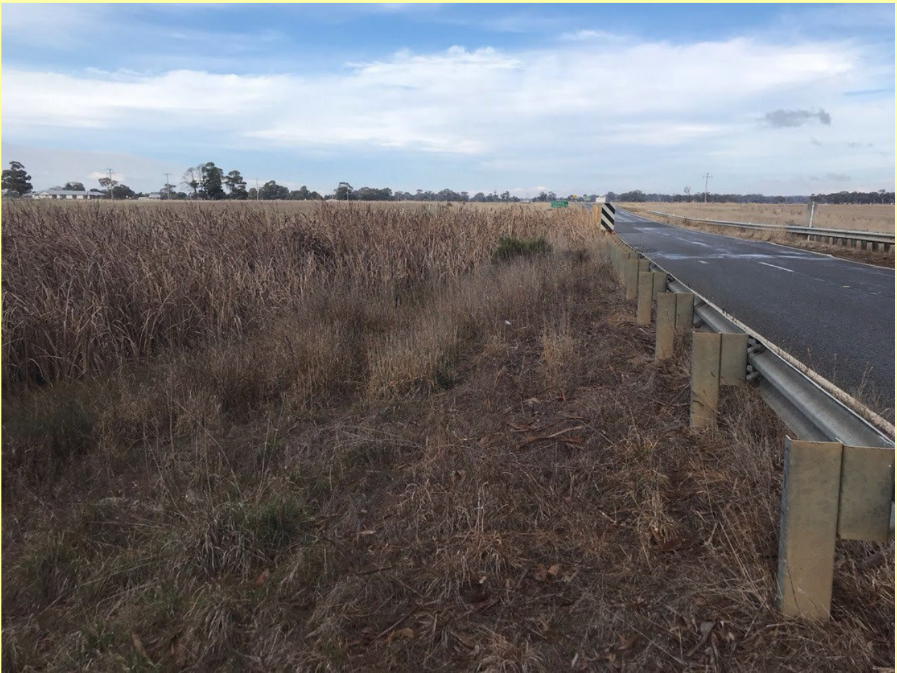
Figure 4-29 Eddington Road Culverts overgrown with Reeds
