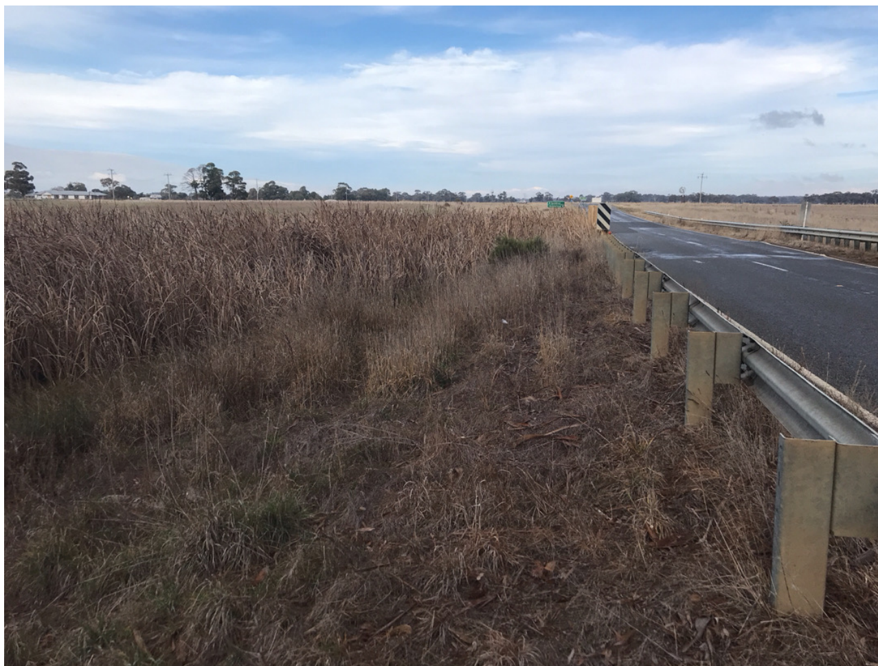
Figure 4-29 Eddington Road Culverts overgrown with Reeds
