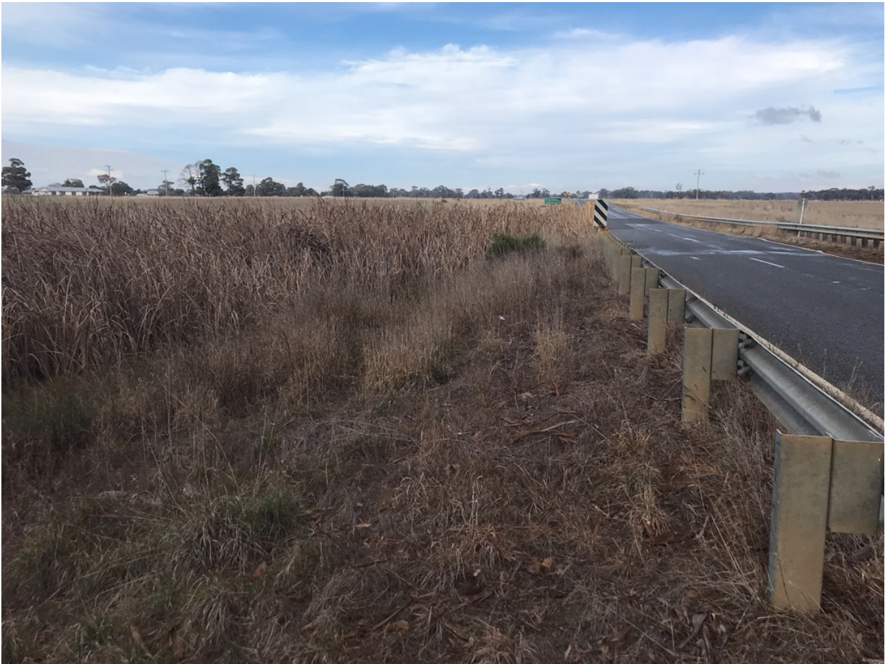
Figure 4-29 Eddington Road Culverts overgrown with Reeds
